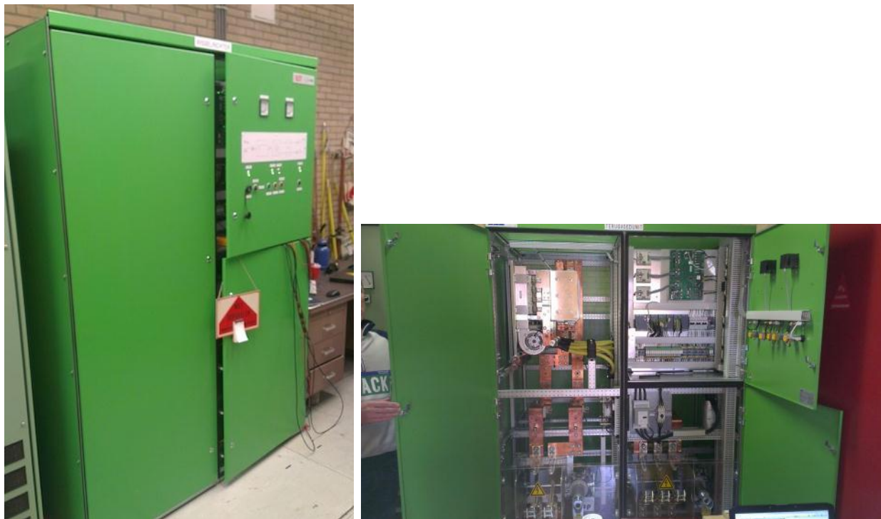
Figure 42: View of the IMTECH inverter
