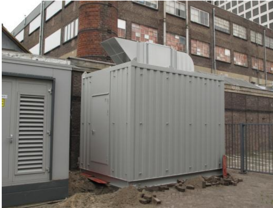
Figure 35: View of the container hosting the supercapacitors storage system, RET
