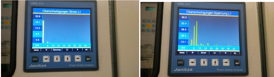
Figure 30: Meter “Janitza” measuring ripple harmonics in substation Oetkerhalle
