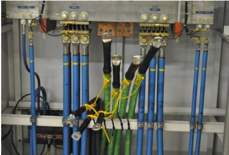
Figure 21: Adaptation of the connections of the high voltage cables to the transformer, STIB
